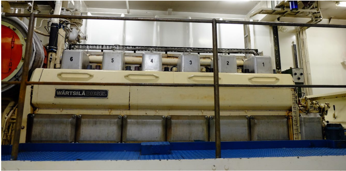
Figure 2. One of two main engines on a diesel-powered car ferry.
